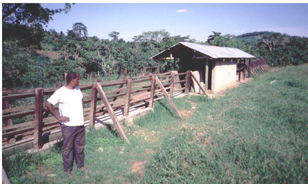
Cattle dip tank. The entrance race, upper walls, rain roof and at far right the draining race are shown.
