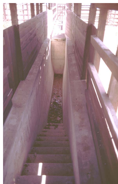
Internal construction of dip tank. Jump off point at far end, deep narrow tank, splash walls and exit steps at near end are shown.
